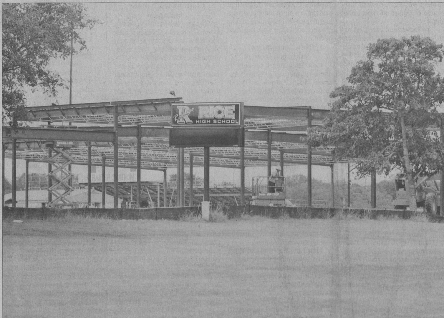
Construction in Altair on the new Junior High Facility is progressing. With the foundation work done, the skeleton of the structure is taking shape. The school is scheduled for completion July 2009, in time for the 2009-2010 school year.
