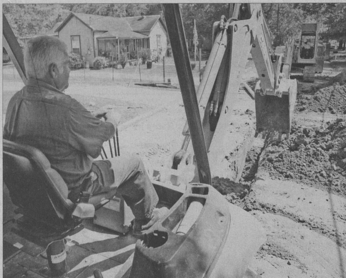
Work continues on Norris Street, where the sewer main is being replaced down the length of the street. The work is being completed as part of a community development block grant.
